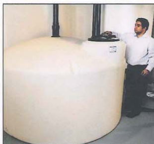
Rahul Kochar adopted a recovery system, which collects rain water from the roof for the five toilets.
